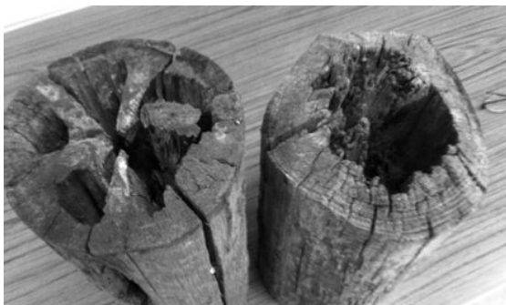
Cross-sections from two of the rotten lighting poles
